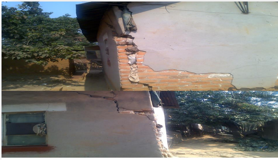
2 Broken houses due to blasting
