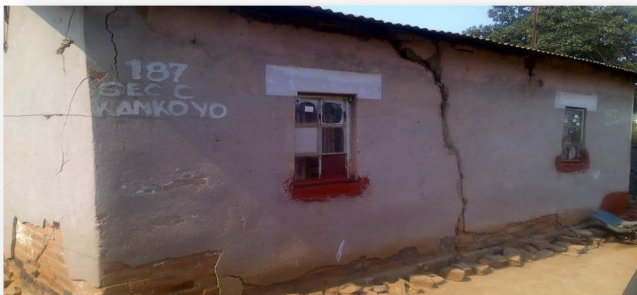
3 Broken houses due to blasting
